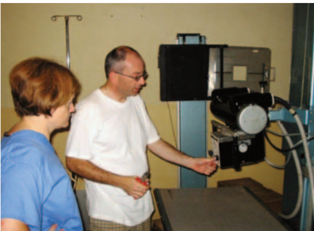
Below: Our electrician assesses the angled tube head and the problem with the light beam diaphragm.
