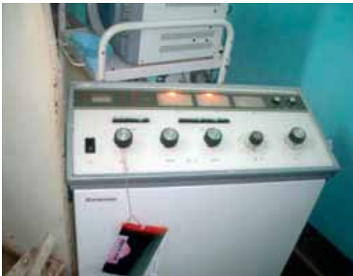
The control panel in the general x-ray room.
